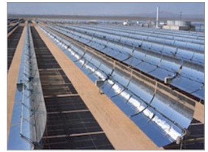
Figure 13.24: Parabolic trough-based ST plant, in which part of the power generation facility is seen in the background. Reflectors must be spaced out to prevent self-shadowing. From U.S. DoE.
